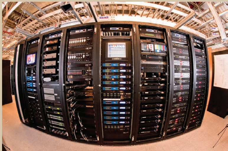
For incoming signals, survivability design dictated multiple antennas in parallel paths for broadcast and satellite sources with impedance-matched utility gain active multicouplers and stacked distribution methodology. Photo by Ron Baker
